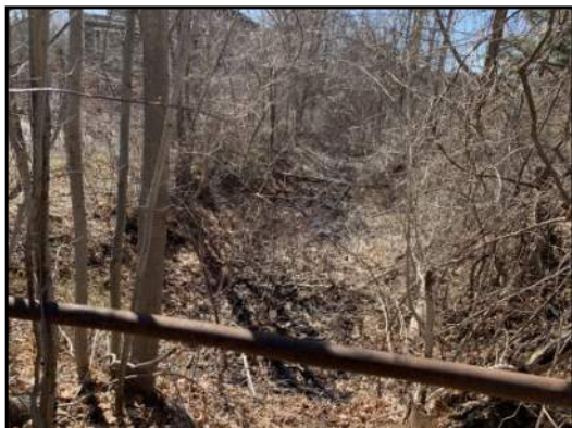
7 : The Mill Race, when flowing, runs to the west to the Mill, beneath the Mill, and discharges to Furnace Creek. View to the west.
