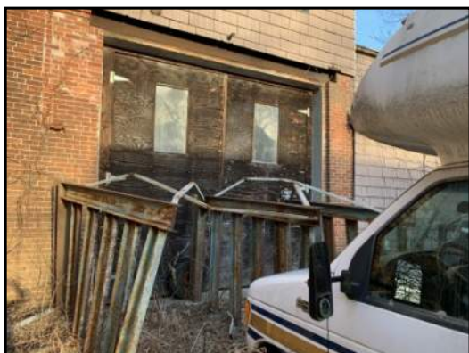
27 : Loading dock off the west side of the Site building. View to east.
