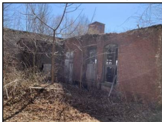
10 : Front (east) side of the former carding portion of the Site building. View to southwest.
