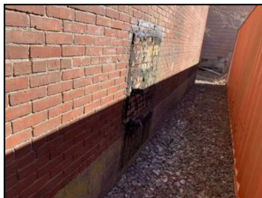
16 : Possible vent/fill pipes for interior AST along the south side of the boiler building.
