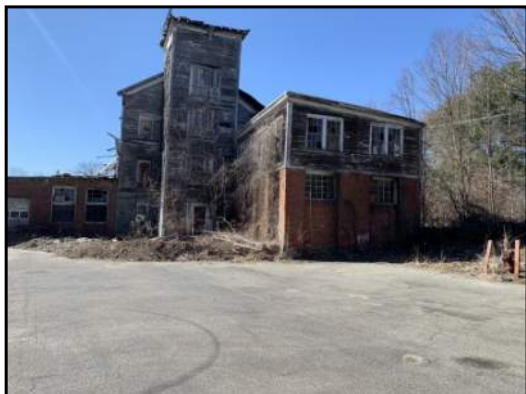
1 : View of the front of the Mill building from the asphalt parking lot. View to the west.
