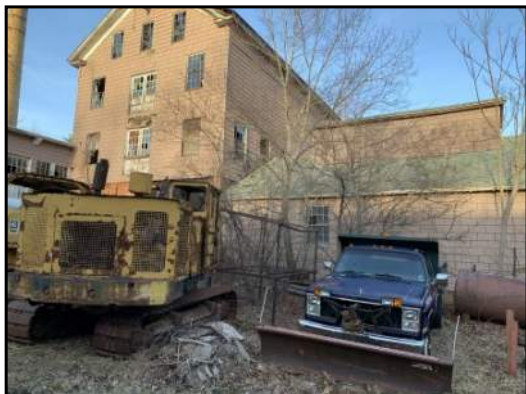
25 : Empty AST (AST #2) along southwest corner of Site building. View to the east.
