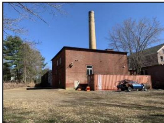
14 : View of the northwest corner of the Site building from adjoining property to the north. View to east-southeast.
