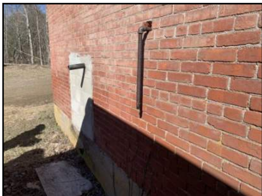
17 : Possible vent pipe for interior AST along the south side of the boiler building. Possible condensate line in foreground. View to the northeast.
